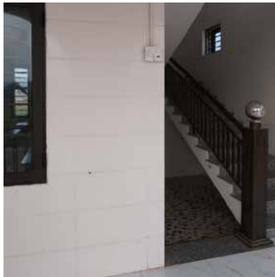
Fig. 34_ Example of elevated electrical installations in a flood prone floor level to adapt to floods (left)
